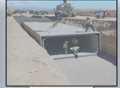
349 miles Storm Drains
